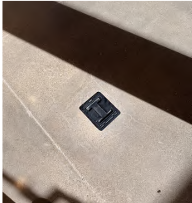
Photo #52: Electrical floor box has wrong cover.
