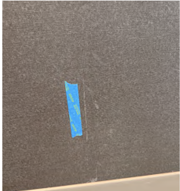
Photo #12: Scratch in wall covering below window into Flight Planning 105
