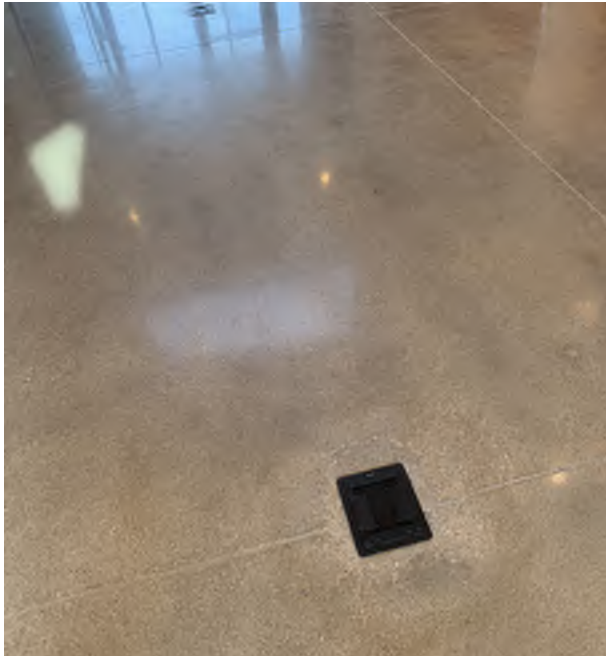
Photo #53: Electrical floor box has wrong cover.
