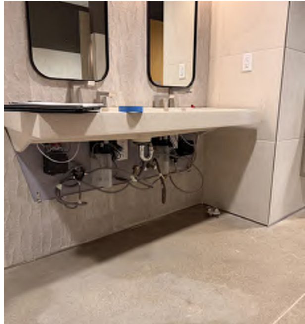
Photo #66: Install missing vanity shroud in Women's 115.
