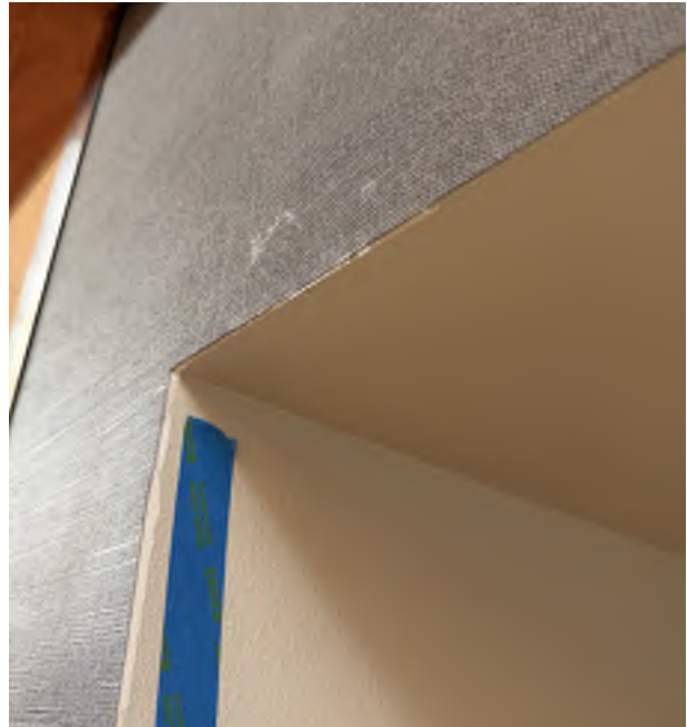
Photo #20: Wall covering fibers along ceiling edge in vending machine alcove.
