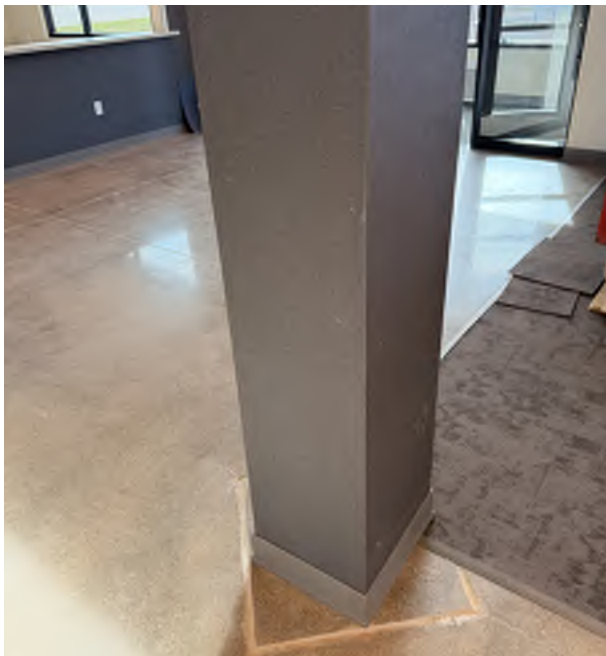
Photo #47: Wall covering shows dirt and adhesive residue throughout. Condition is consistent across all wall covering locations.
