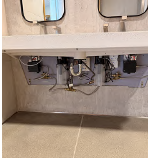
Photo #54: Install missing vanity shroud in Men's 114.
