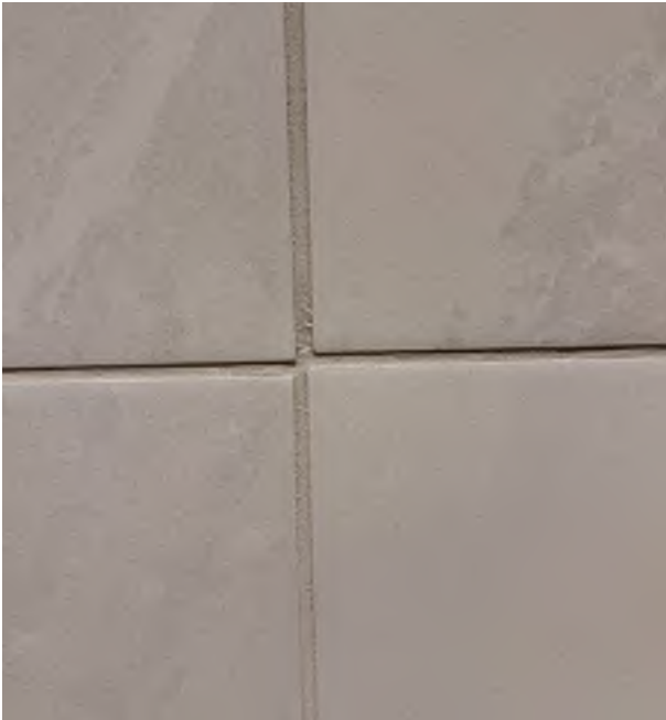
Photo #67: Wall tile installation exhibits multiple workmanship deficiencies. Lippage and misaligned tiles pictured above.
