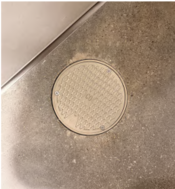
Photo #71: Provide sealant around cleanout assembly. Typical at all locations.
