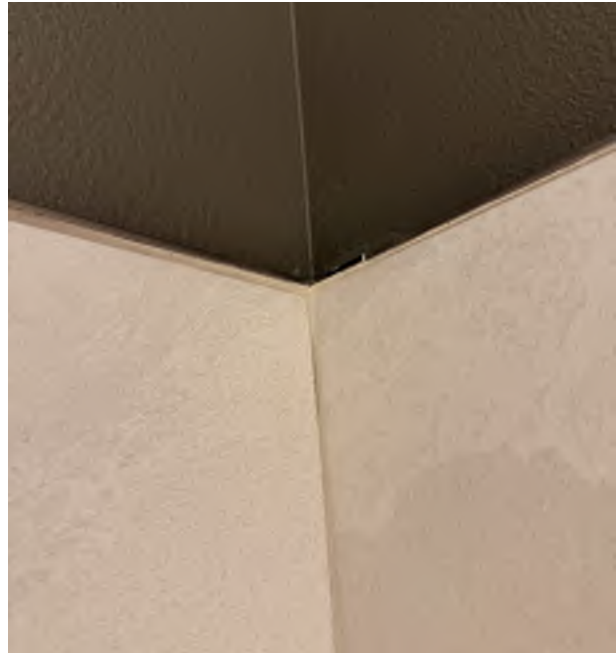
Photo #68: Wall tile installation exhibits multiple workmanship deficiencies. Misaligned tiles pictured above.
