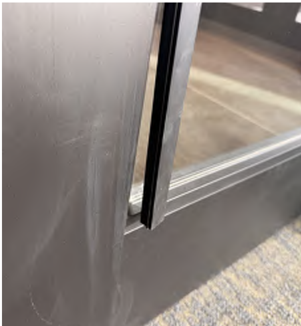
Photo #31: Glazing stop hanging off Door 110C
