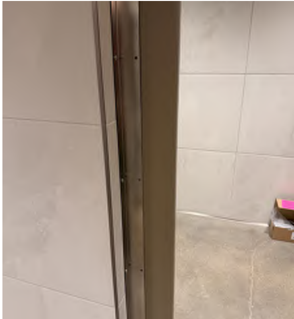
Photo #73: Toilet partition is missing screws in Women's 115
