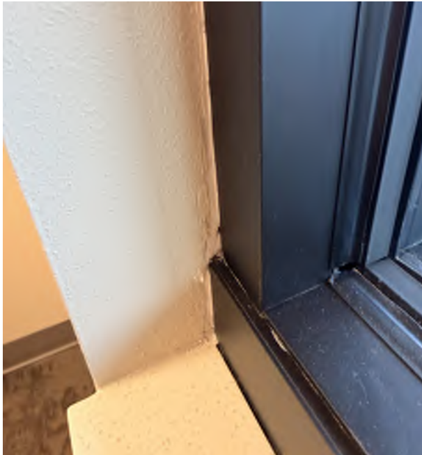
Photo #23: Exterior window frame and wall joint looks unfinished and rough. Condition is consistent across all exterior window locations. Missing sealant at joint between window frame and window sill.
