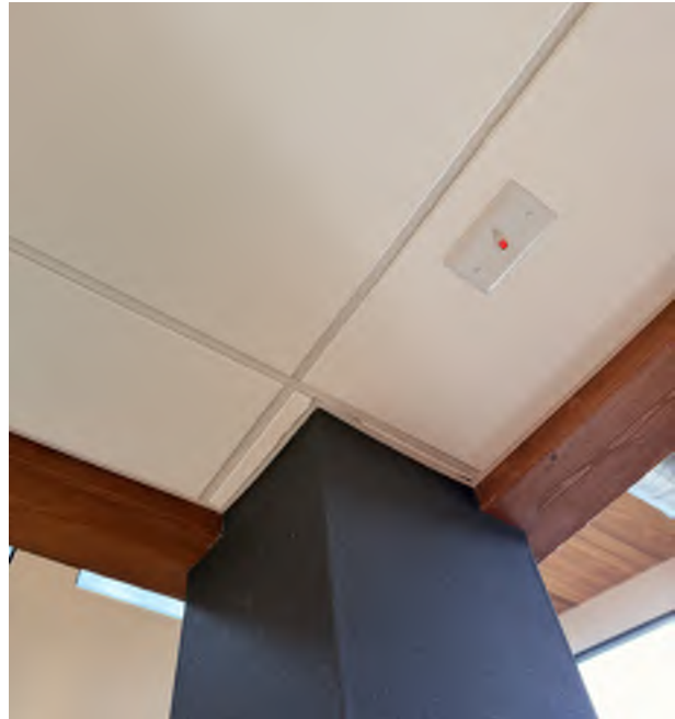
Photo #46: Ceiling around column in Kitchenette 112 includes undersized ACT border pieces, not in compliance with specifications.
