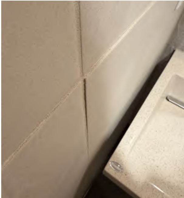
Photo #59: Wall tile installation exhibits multiple workmanship deficiencies. Lippage pictured above.
