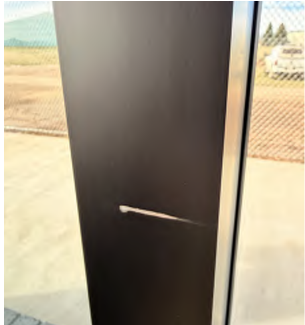
Photo #38: Scuffed wall base
