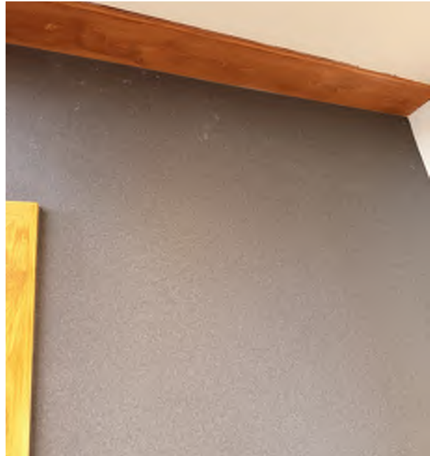
Photo #8: Wall covering shows dirt and adhesive residue throughout. Condition is consistent across all wall covering locations.
