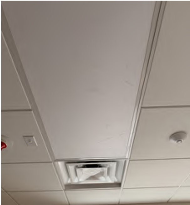
Photo #29: Dirty light fixtures in Control 108
