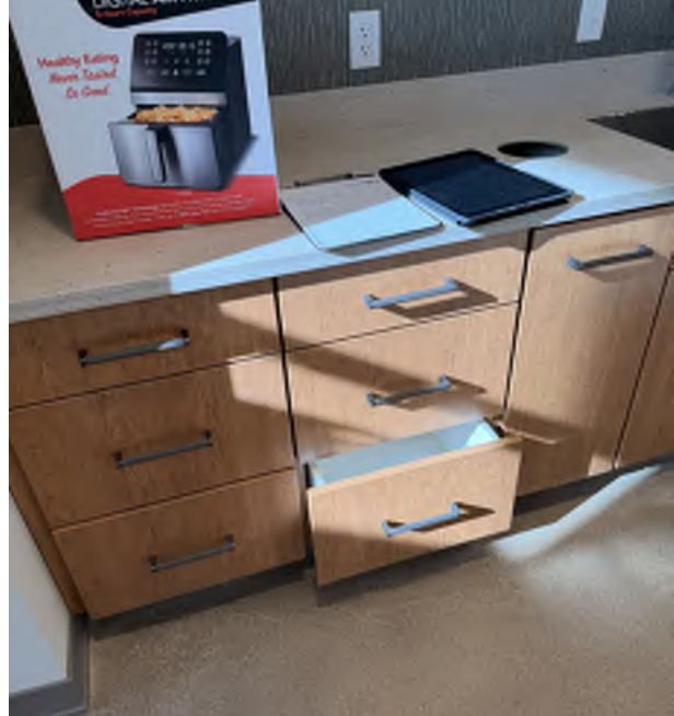
Photo #50: Open drawer pictured in Kitchenette 112 needs adjustment.
