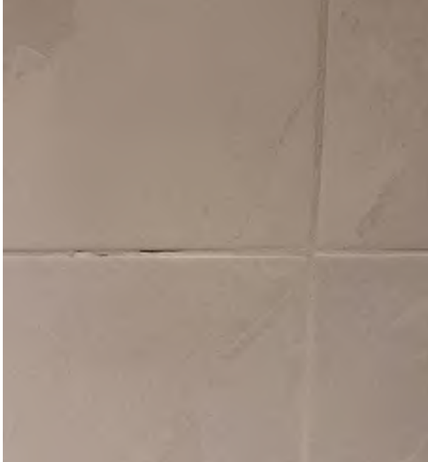
Photo #57: Wall tile installation exhibits multiple workmanship deficiencies. Misaligned tiles and uneven grout join pictured above.
