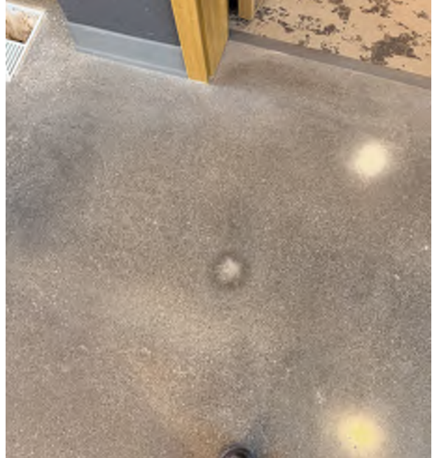
Photo #18: Exposed concrete shows irregularities and/or stains. Contractor to verify condition and coordinate corrective action as required.
