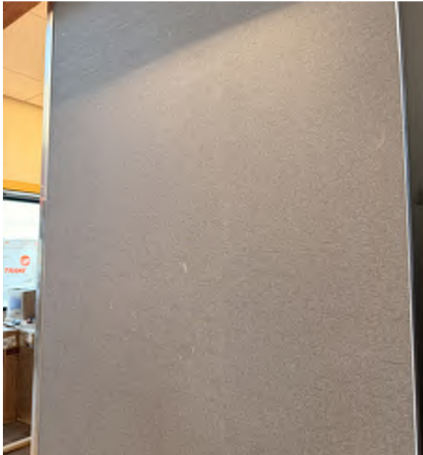
Photo #11: Wall covering shows dirt and adhesive residue throughout. Condition is consistent across all wall covering locations.
