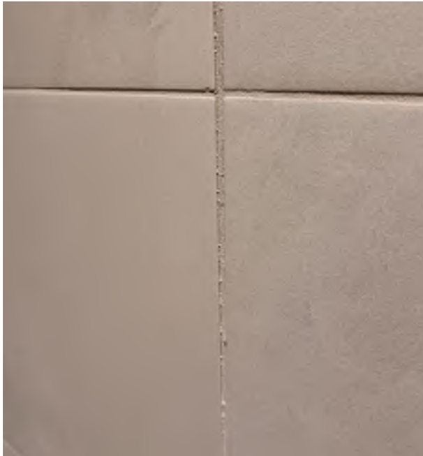
Photo #63: Wall tile installation exhibits multiple workmanship deficiencies. Lippage and uneven grout joint pictured above.
