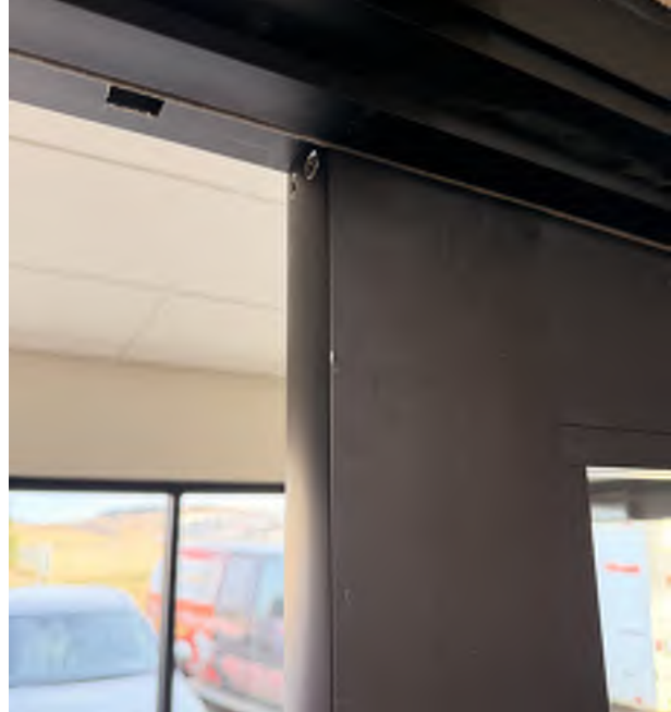
Photo #2: Scratches on Door 100B
