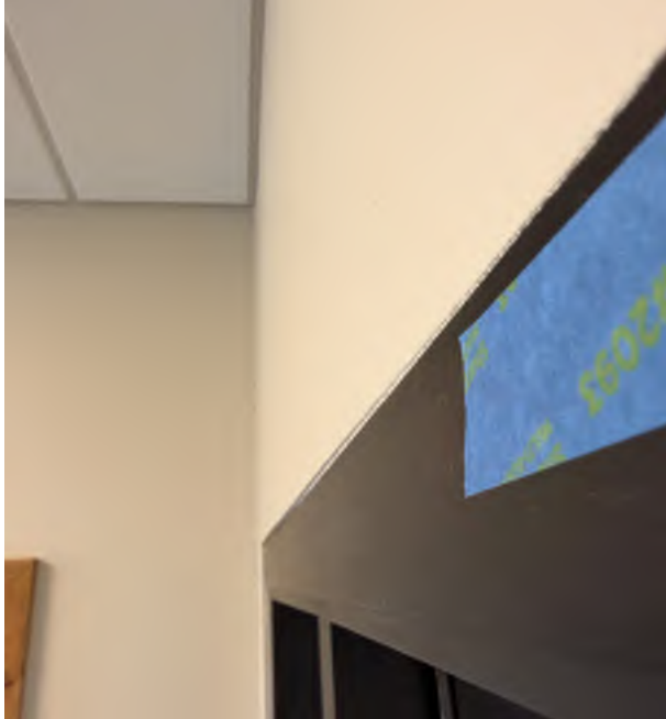
Photo #25: Door 106B frame is inconsistently aligned with adjacent wall surface – flush in some areas and projecting in others.
