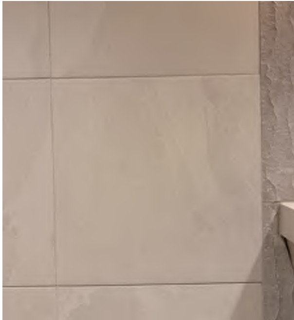
Photo #65: Wall tile installation exhibits multiple workmanship deficiencies. Lippage and uneven grout joint pictured above.
