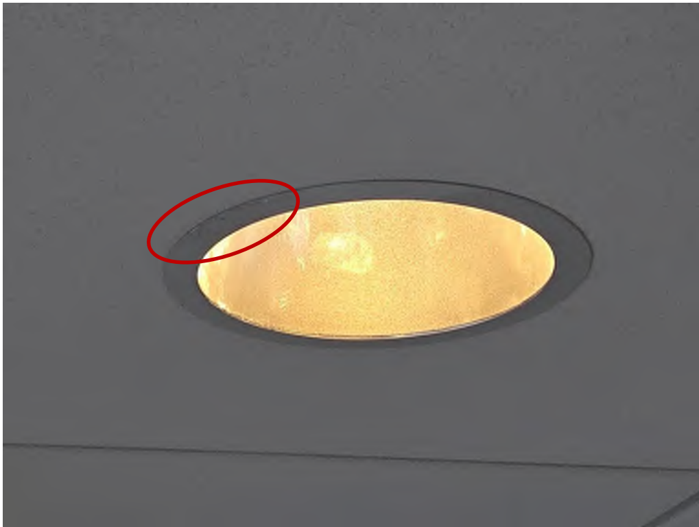
Vestibule 100 Damaged Trim
