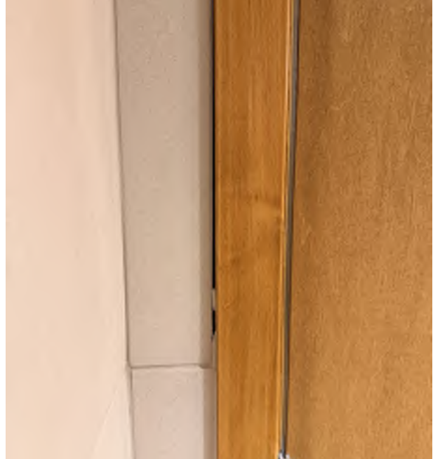
Photo #58: Exposed gap on hinge side of Door 114.
