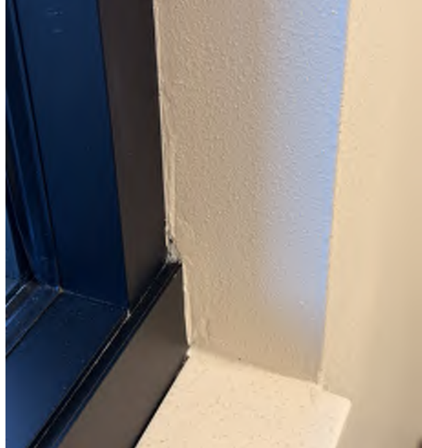
Photo #22: Exterior window frame and wall joint looks unfinished and rough. Condition is consistent across all exterior window locations.
