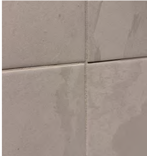
Photo #64: Wall tile installation exhibits multiple workmanship deficiencies. Lippage and uneven grout joint pictured above.
