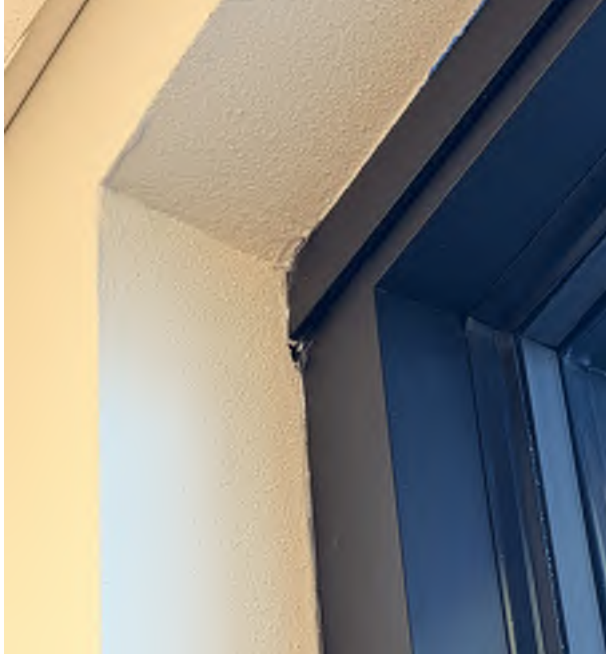
Photo #21: Exterior window frame and wall joint looks unfinished and rough. Condition is consistent across all exterior window locations.
