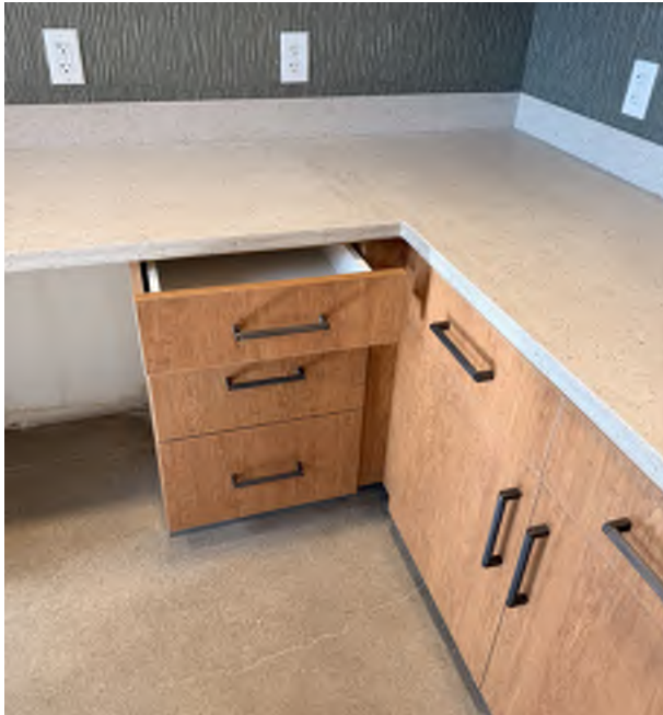
Photo #51: Open drawer pictured in Kitchenette 112 needs adjustment.
