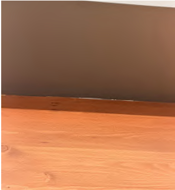
Photo #9: Messy joint at glulam to light shelf
