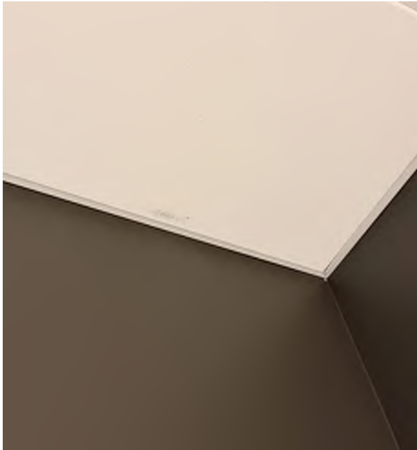
Photo #69: Scuffed ceiling tile in Women's 115.
