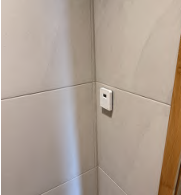
Photo #61: Wall tile installation exhibits multiple workmanship deficiencies. Small sliver of tile used in corner instead of balancing tile layout on wall.
