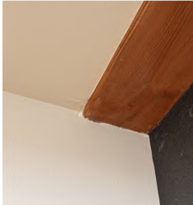
Photo #4: Glulam to wall joint above Door 100B is rough and incomplete - visible gaps, uneven drywall, and unpainted areas.
