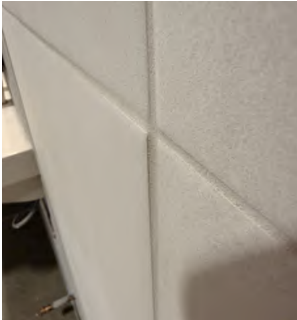
Photo #55: Wall tile installation exhibits multiple workmanship deficiencies. Lippage pictured above.
