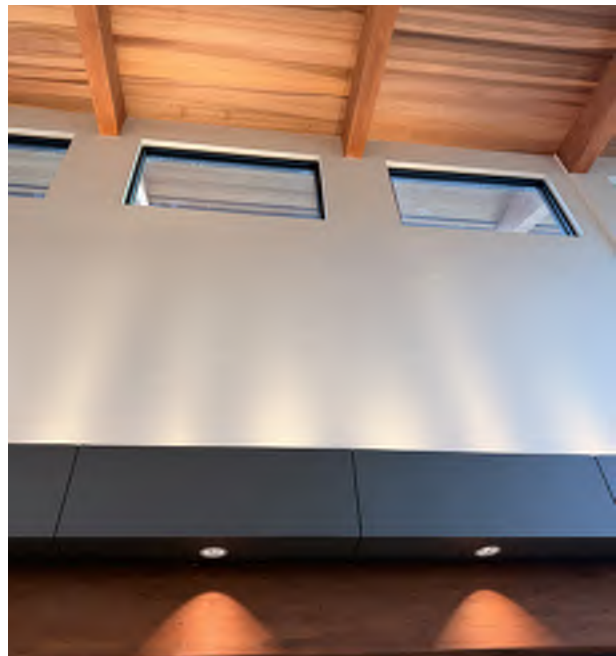
Photo #16: Aimable spot lights on top of light shelf need to be directed to centerline of the Concourse, not directly up. Windows are also dirty.
