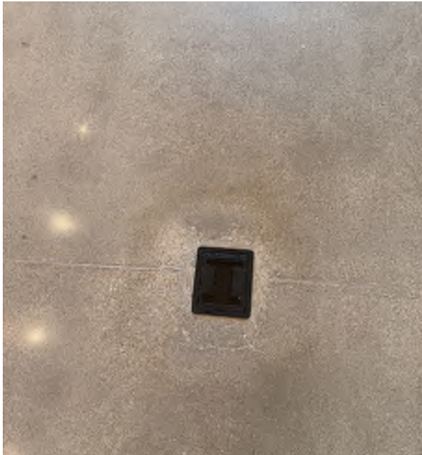
Photo #19: Electrical floor box has wrong cover.
