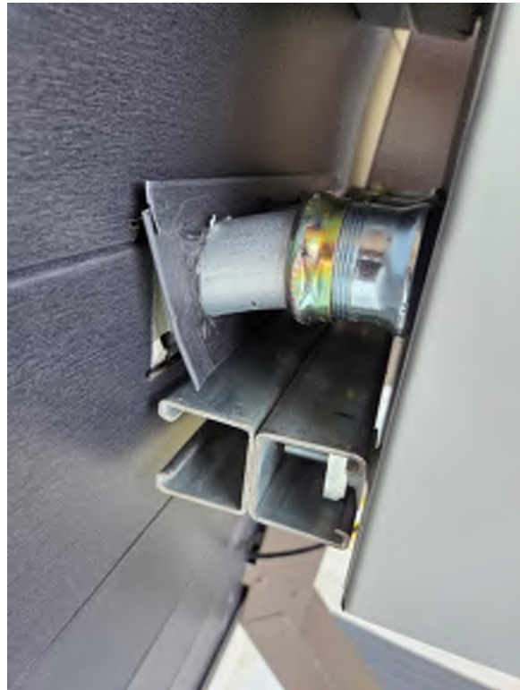
Comms J-Box on Roof – Needs Sealed
