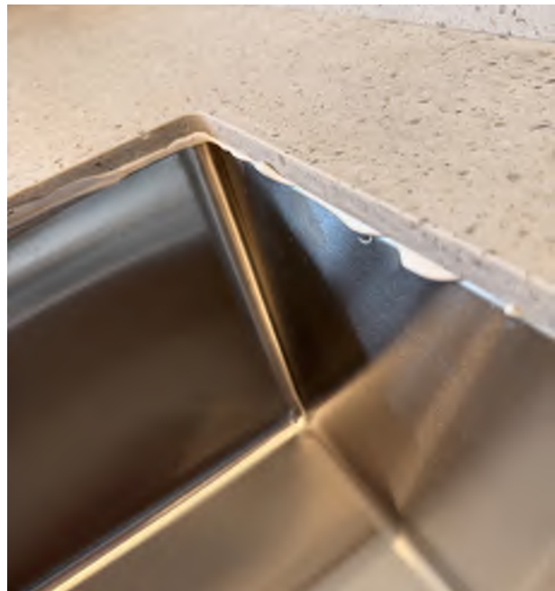
Photo #48: Caulk is exposed at undermount sink in Kitchenette 112
