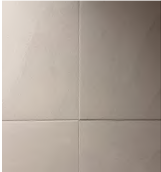
Photo #70: Wall tile installation exhibits multiple workmanship deficiencies. Lippage and uneven grout joint pictured above.
