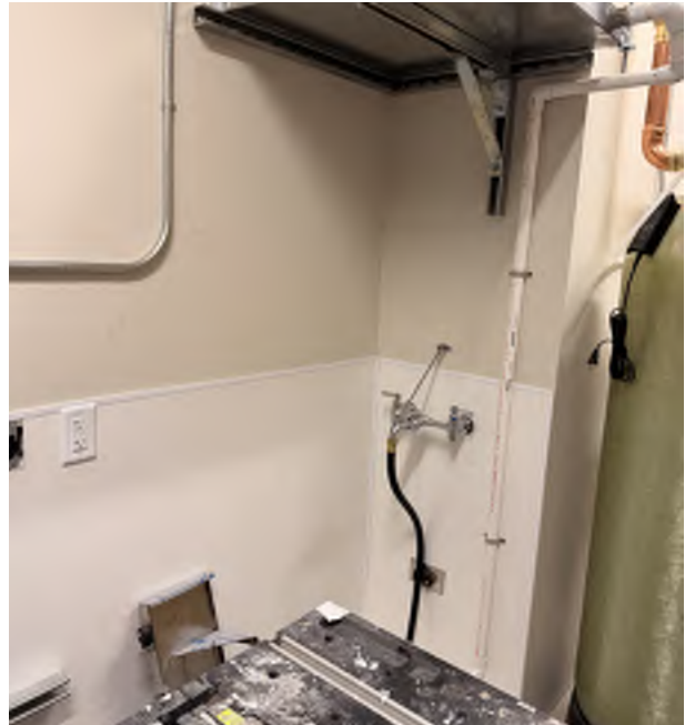
Photo #76: Install missing utility shelf in Utility 117.
