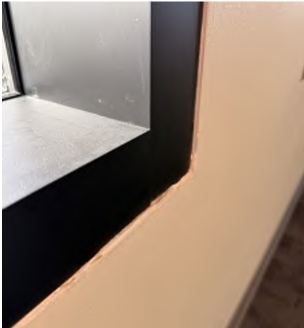
Photo #43: Curtain wall framing exhibits inconsistent alignment relative to adjacent wall assemblies – recessed, flush, and projecting conditions observed. Condition is consistent across all curtain wall locations.
