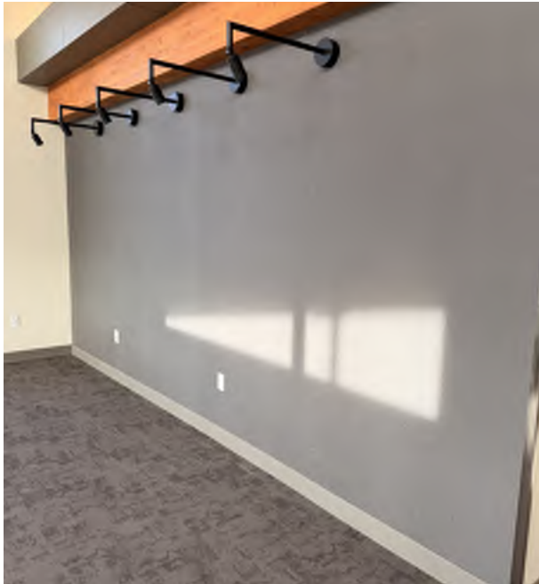
Photo #45: Wall covering shows dirt and adhesive residue throughout. Condition is consistent across all wall covering locations.
