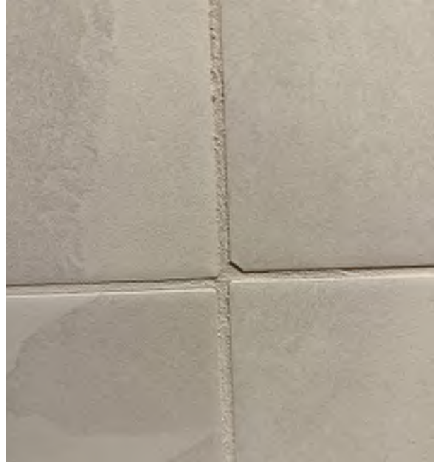
Photo #62: Wall tile installation exhibits multiple workmanship deficiencies. Chipped tile and misaligned tiles pictured above.
