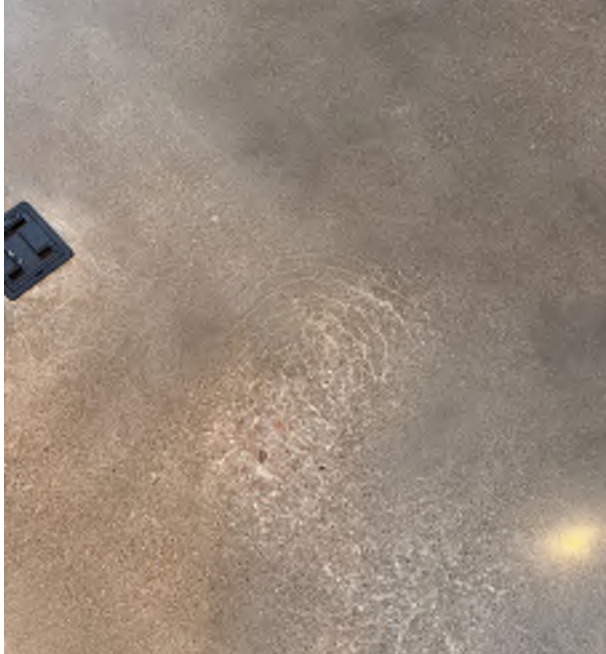
Photo #17: Exposed concrete shows irregularities and/or stains. Contractor to verify condition and coordinate corrective action as required.
