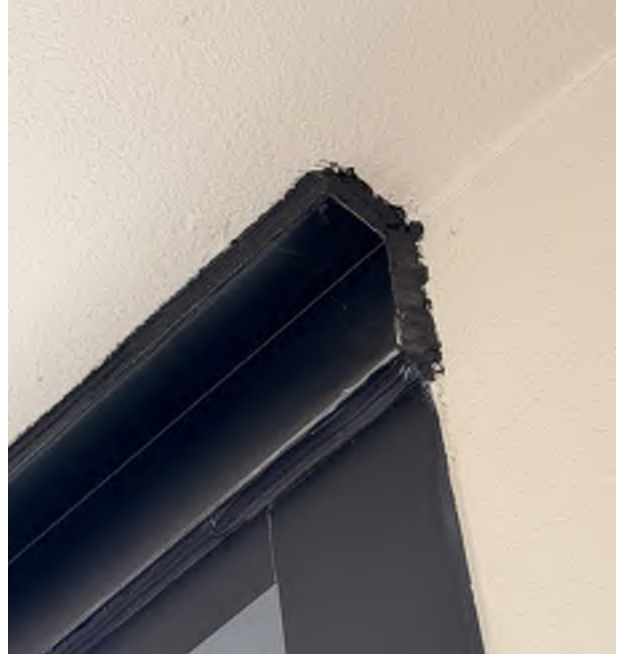
Photo #34: Scuffed wall base
