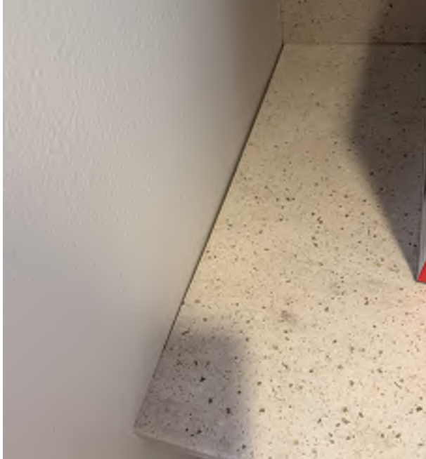
Photo #49: Missing sealant between wall and countertop in Kitchenette 112.
