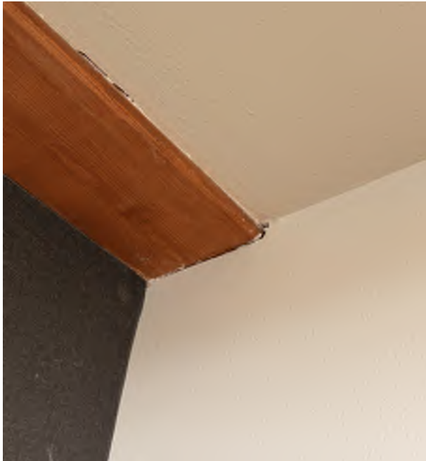
Photo #5: Glulam to wall joint above Door 100B is rough and incomplete - visible gaps, uneven drywall, and unpainted areas.
