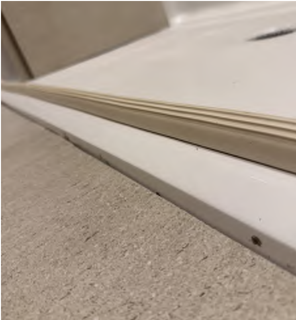
Photo #75: Tile floor transition to shower is not within acceptable ADA height transition limit.
