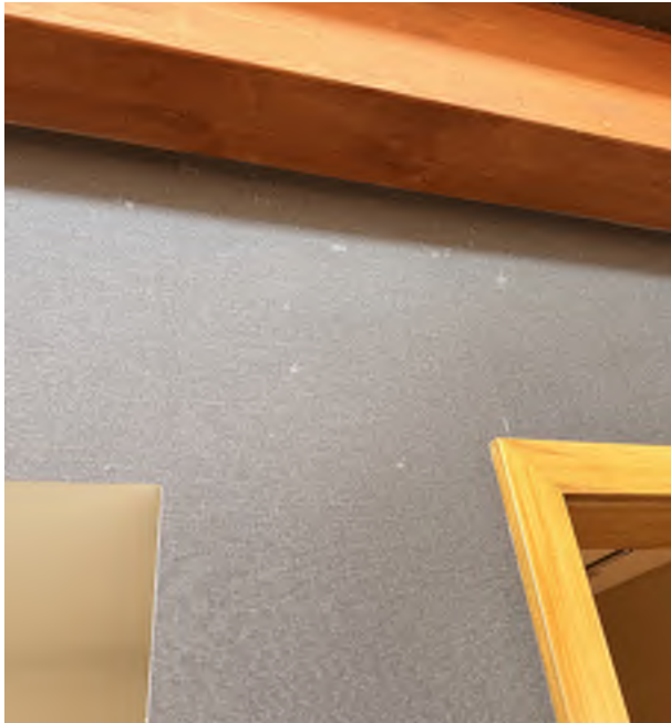
Photo #7: Wall covering shows dirt and adhesive residue throughout. Condition is consistent across all wall covering locations.
